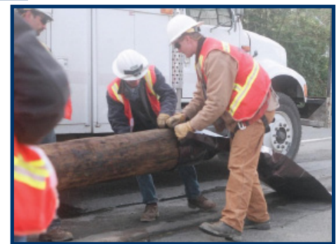
The Field Liner takes just a few minutes to install in the field, immediately prior to setting the pole.
